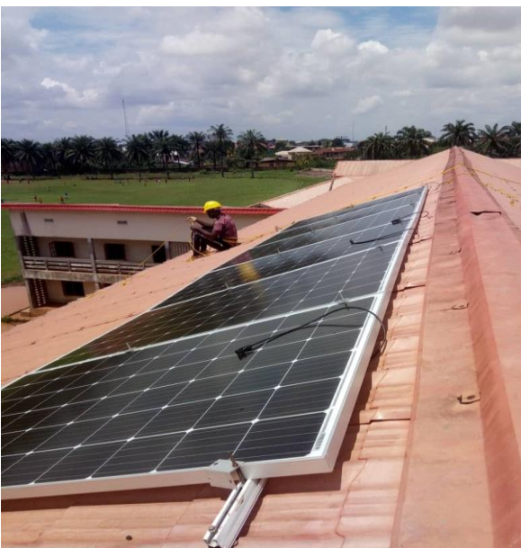
New solar inverter/panels and batteries for the Library
